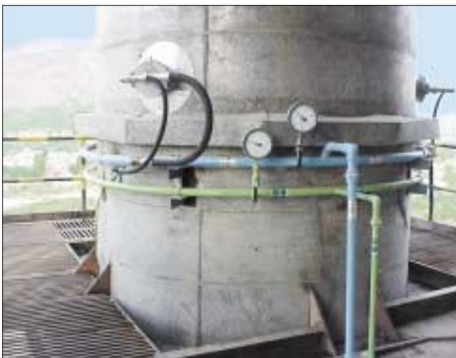
Duct cooling with twin fluid nozzle lances
