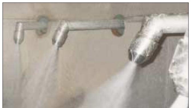
Inside view gas cooling tower
