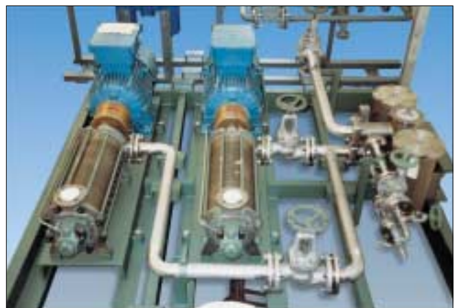
Pump arrangement on a unit
